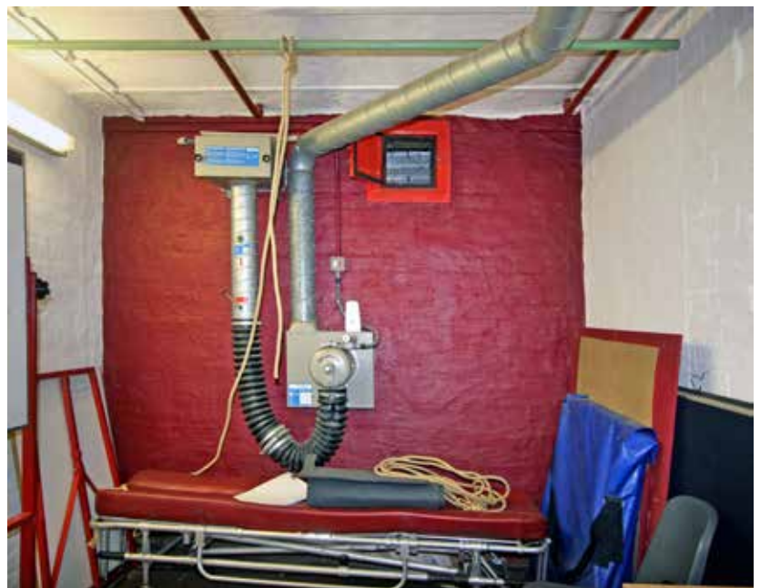
Ventilation plant at the rear of the Fire Brigade room
